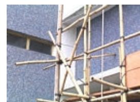
Fig. 1.5 Detail of a putlog attaching the post of the outer layer in a DLBS
