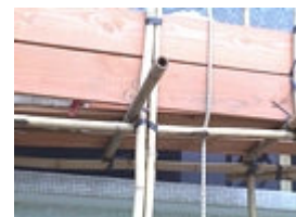
Fig. 1.4 A close-up on the ledger-post connection
